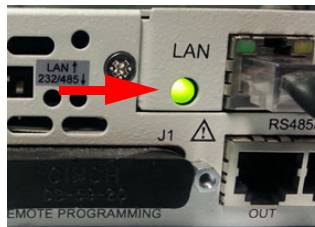
Fig. 6-9 External Power Supply - LAN LED Active
